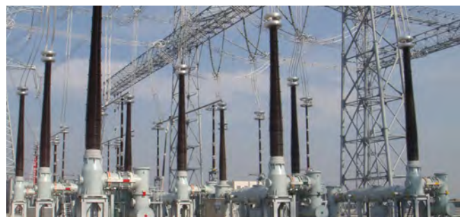
超々高電圧ガス絶縁開閉装置:UHV GIS (Ultra High Voltage Gas Insulated Switchgear)
